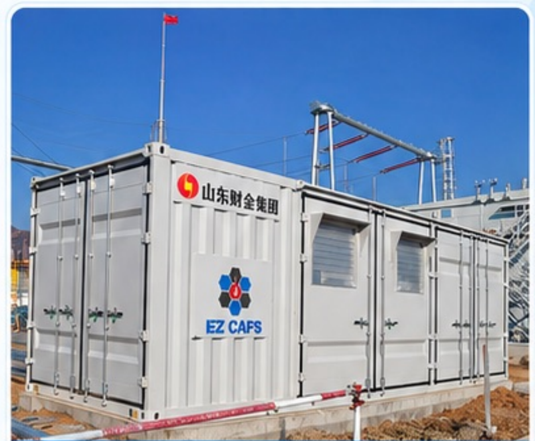
REAL-WORLD INSTALLATION Fixed CAFS container deployed in an industrial site
